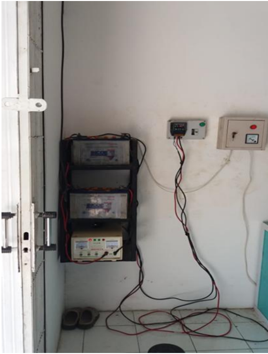
Gambar 2. Ruang Rangkaian Panel Surya
